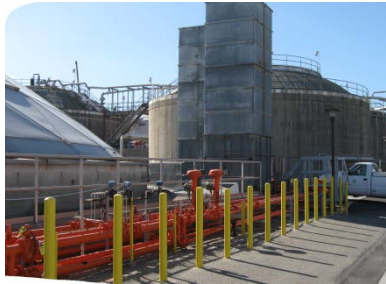
High pressure digester gas waste flare station
